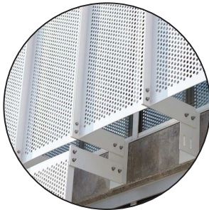
Shade screen to reduce direct sunlight
