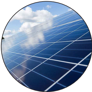
Solar panels on the roof
