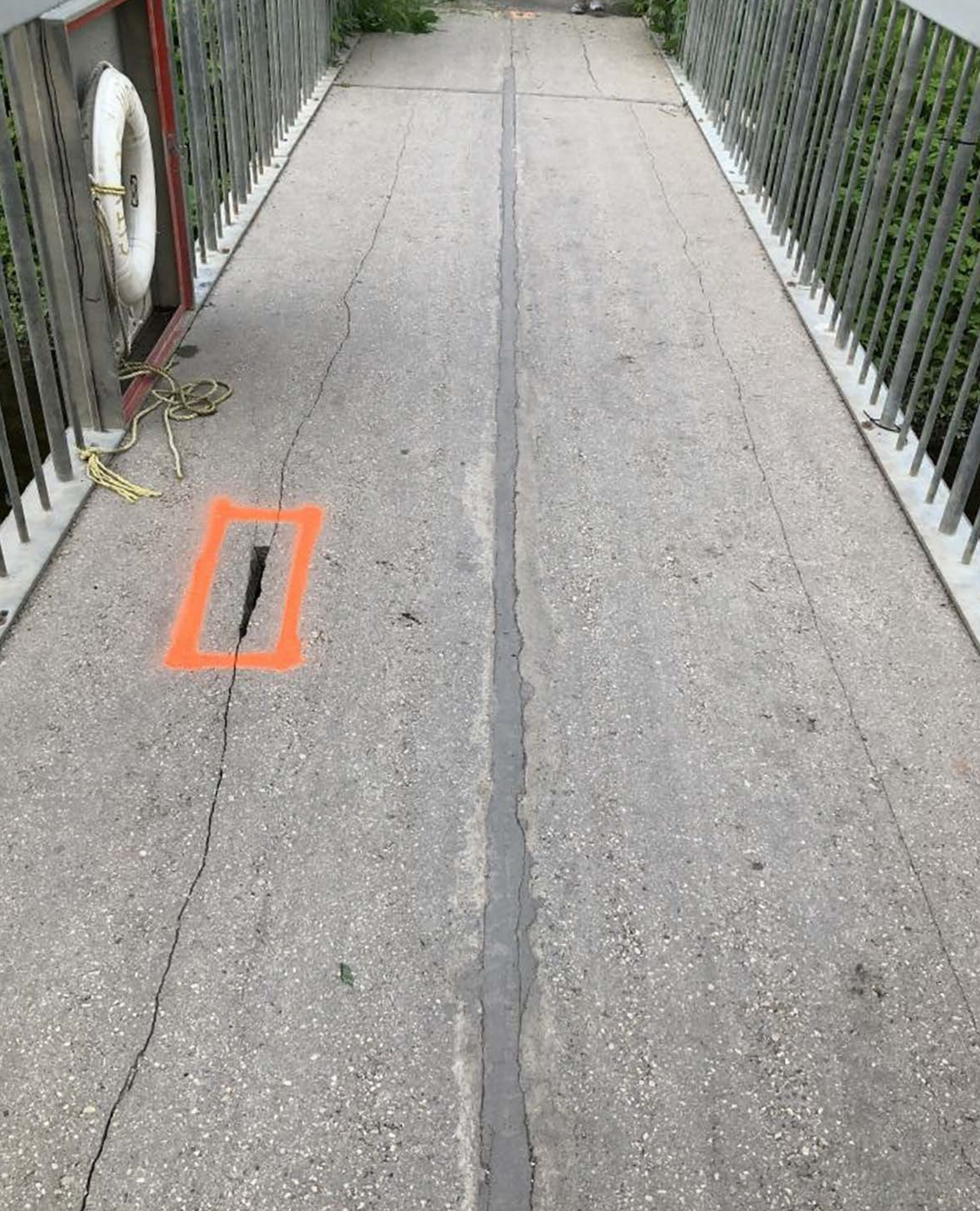
Top of Omand Park pedestrian bridge. Cracks to bridge deck. Taken July 17, 2019x
