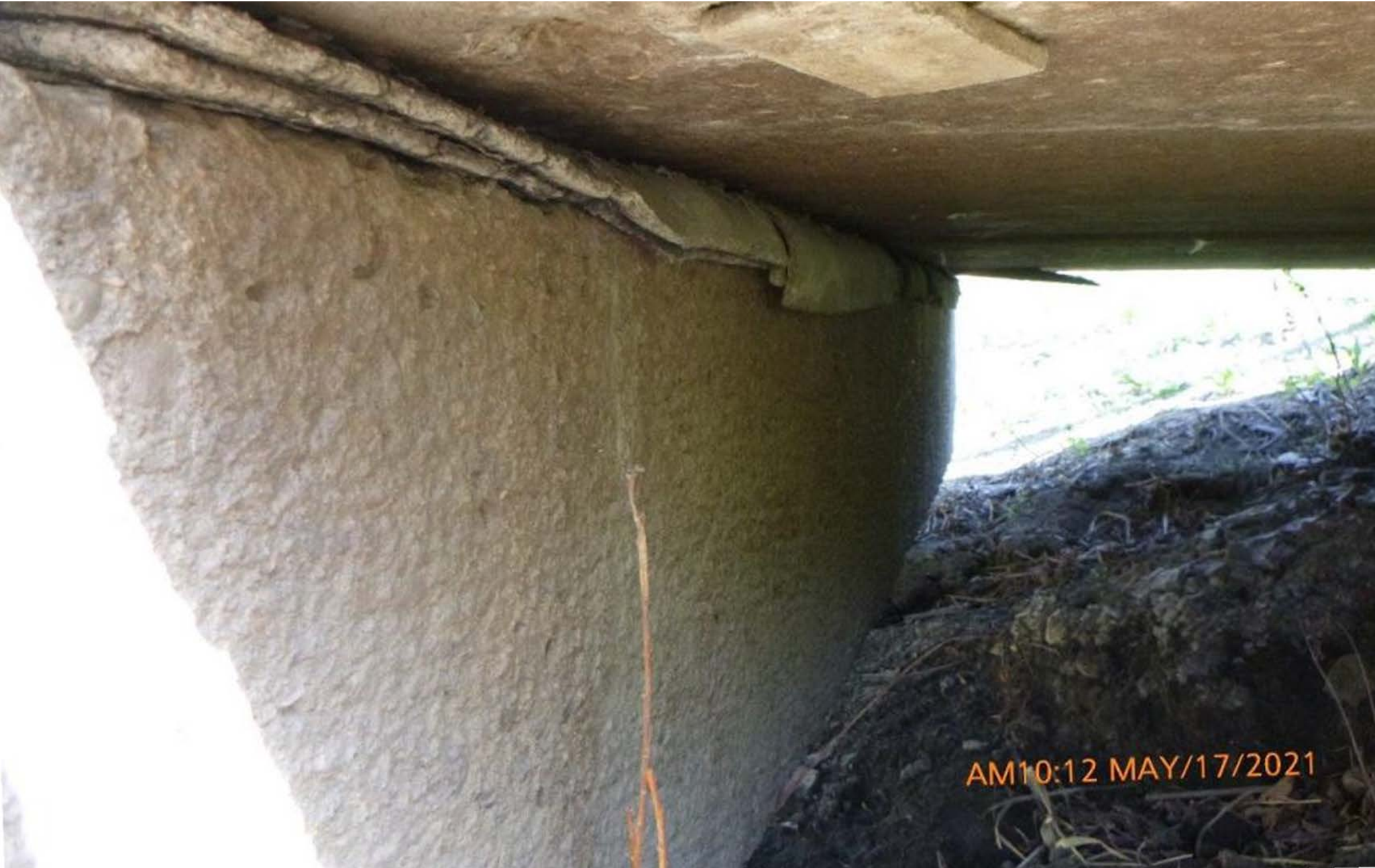
East pier of Omand Park pedestrian bridge. Bulging in bearings. Taken May 17, 2021
