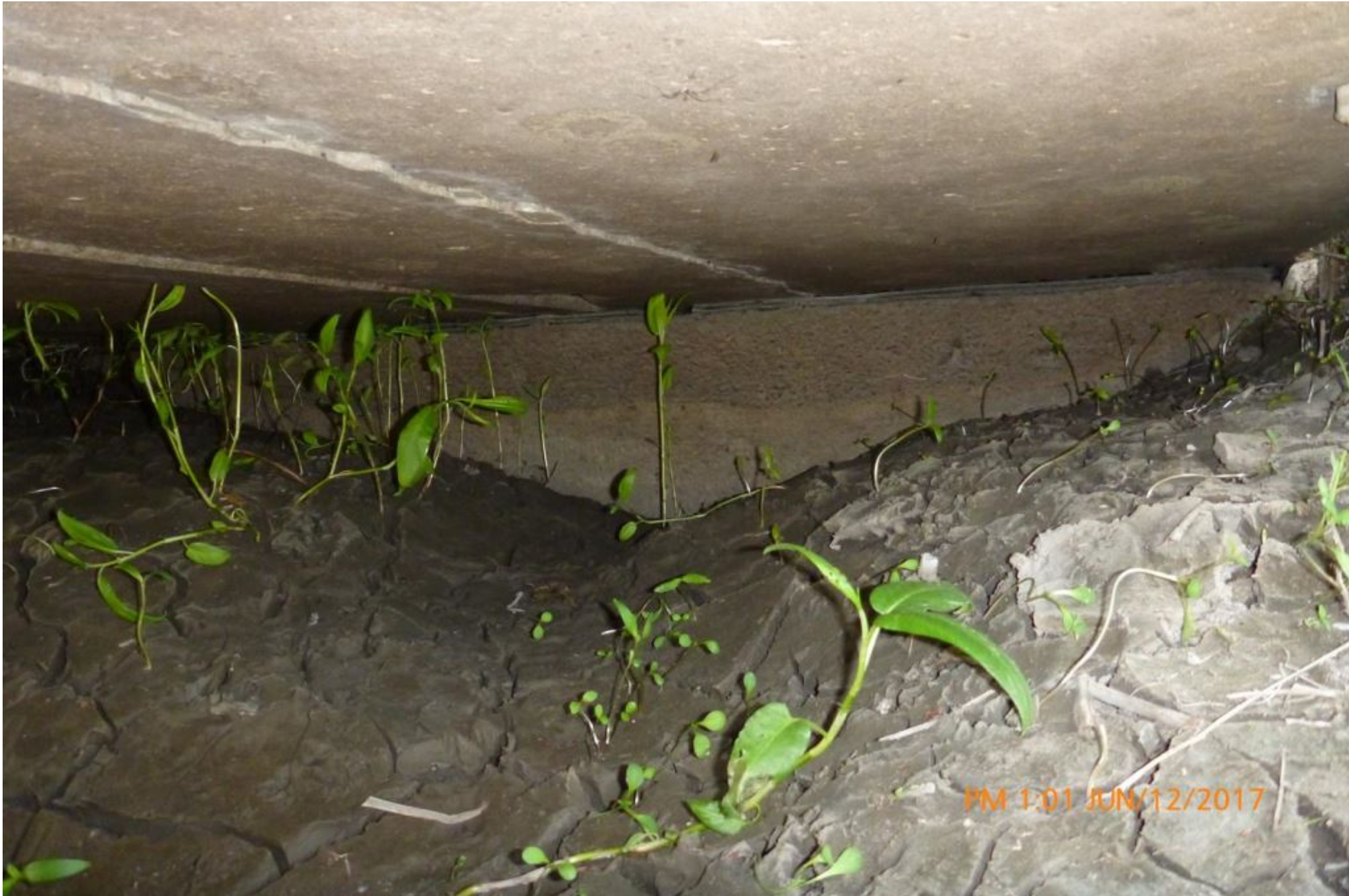
Underside of Omand Park pedestrian bridge. Cracks to bridge deck. Taken June 12, 2017
