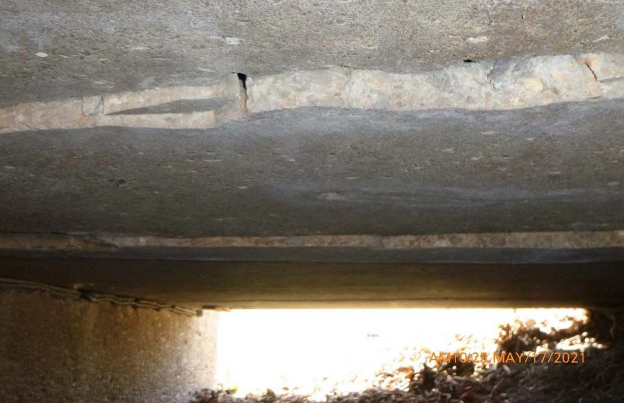
Underside of Omand Park pedestrian bridge. Separation of bridge deck. Taken May 17, 2021
