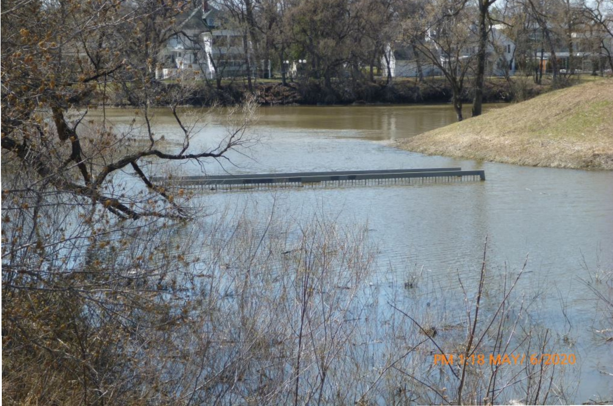
The Structure is Fully Submerged/Flooded. Taken May 6, 2020
